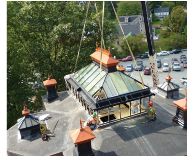
Looking up at the skylight inside the St. Johnsbury Athenaeum. The skylight, glazed with EC glass, protects one of America's most beloved paintings from fading. Bottom photo shows the skylight, replicated to match the Victorian style of the museum, being set onto the roof.
